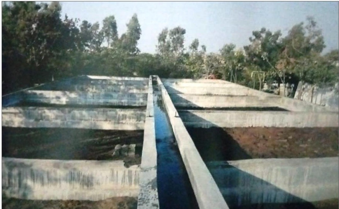
Sludge Drying Beds
