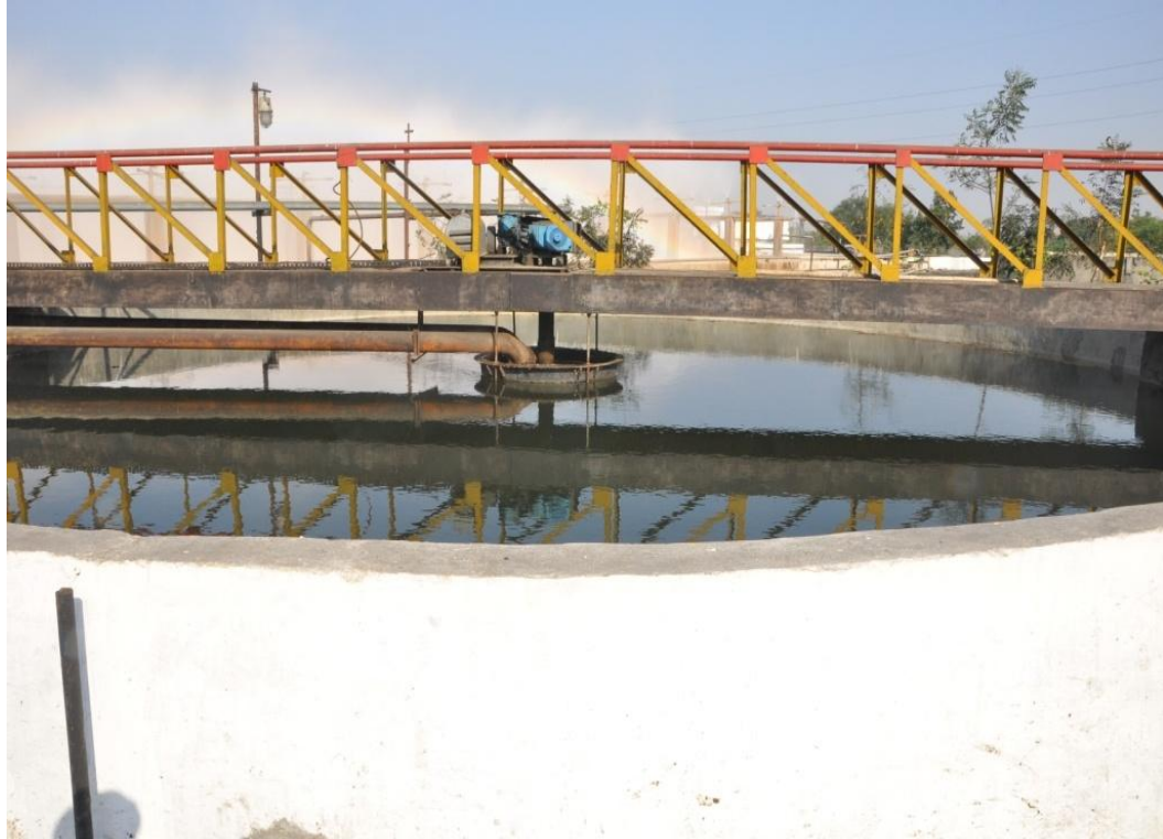
Secondary Clarifier Tank
