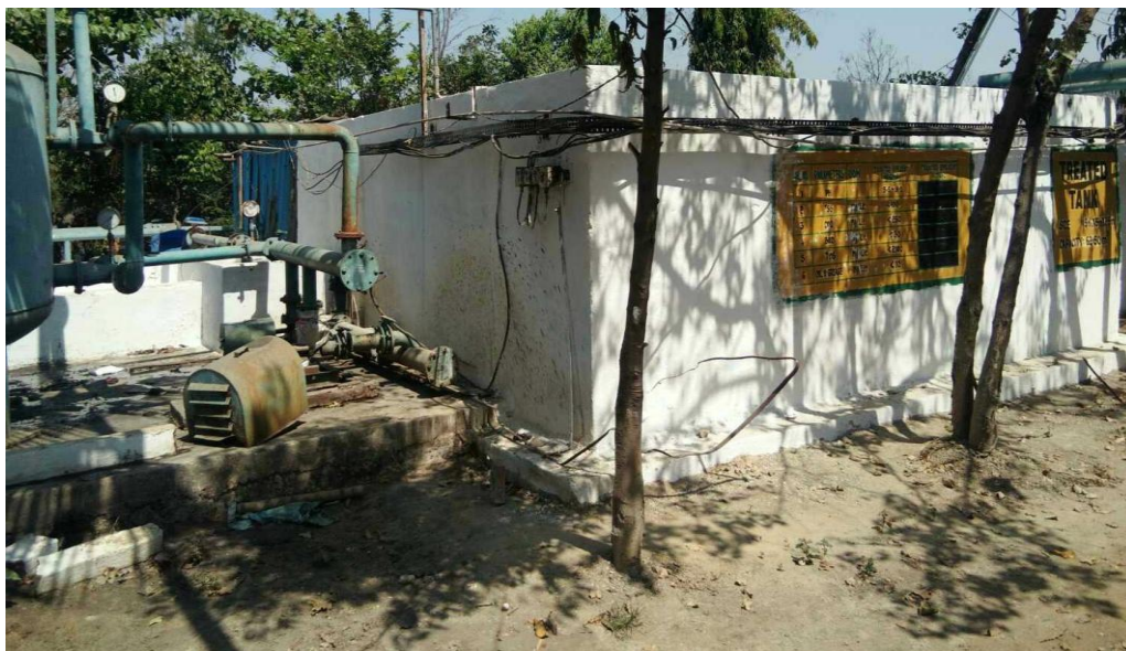
Treated Water Tank
