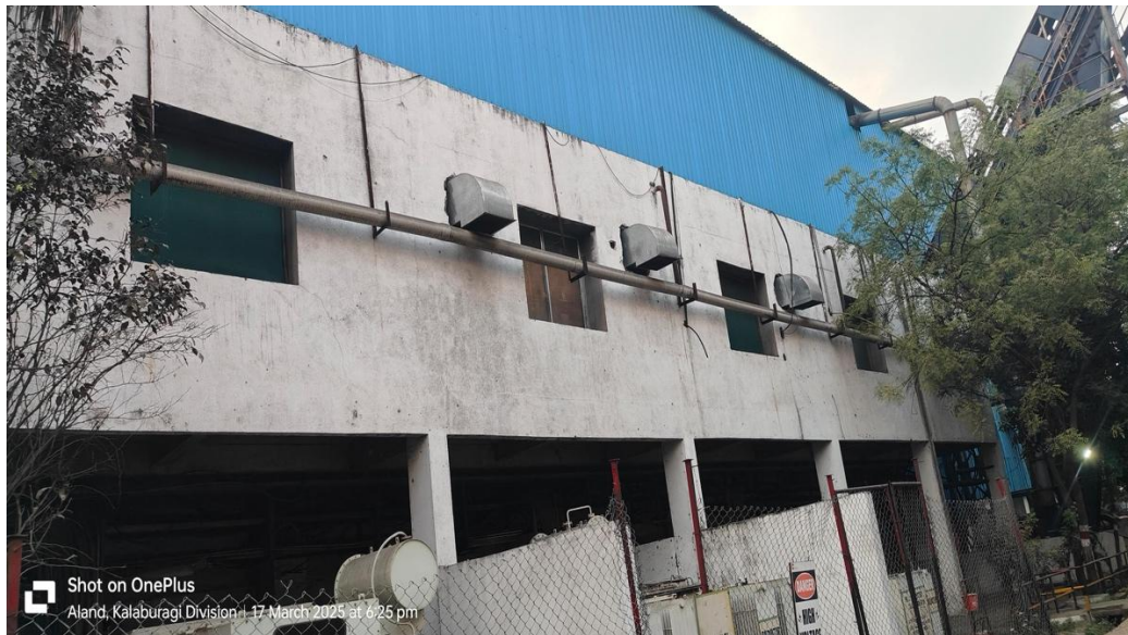
Figure 20: Pipeline arrangement for Rooftop harvesting in Aland unit
